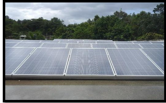
Rock Hall All Age School, St. Andrew - Rainwater Harvesting System Solar Panels Array
