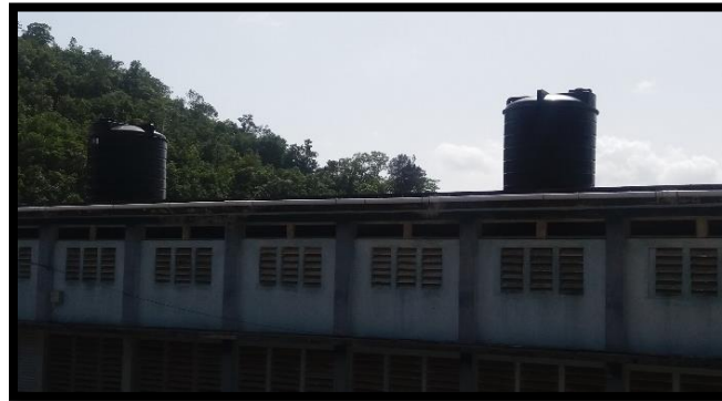
Rock Hall All Age School, St. Andrew (Gravity Feed Distribution Tanks)
