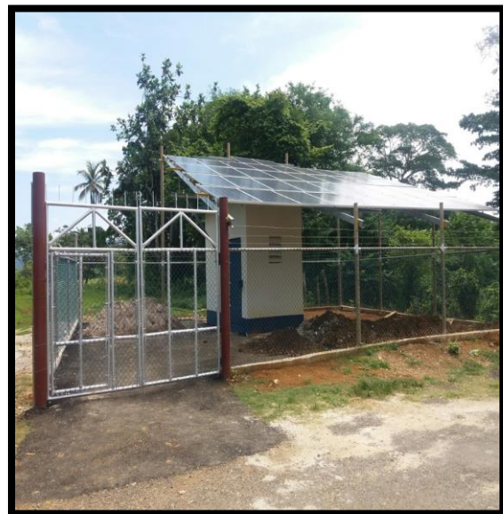
Top Reading Water Supply System, St. Elizabeth - Pump House with Solar Panel Array
