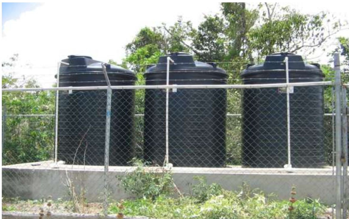
Hill Sixty Roto-Plastic Storage Tanks.
