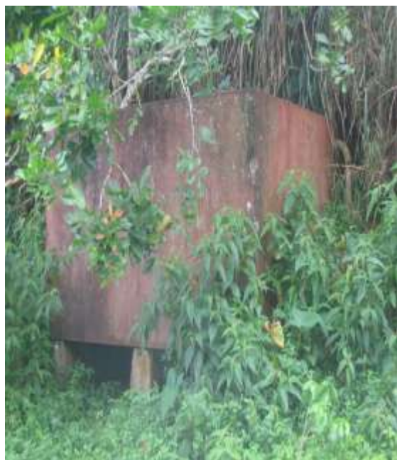
Waugh Hill Relift Pump Feeder Tank - Before
