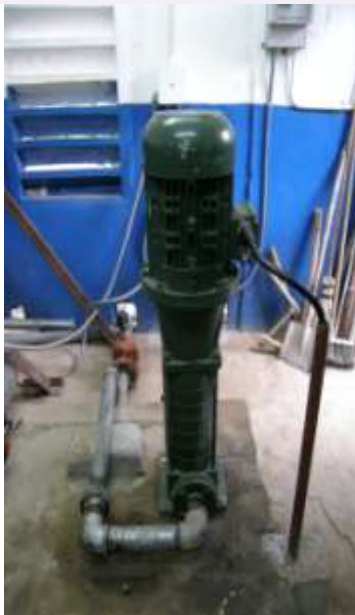
James Hill Water Supply: Vertical Pump
