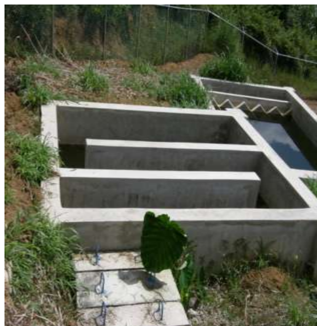
Cascade Water Supply : Flocculation Tank
