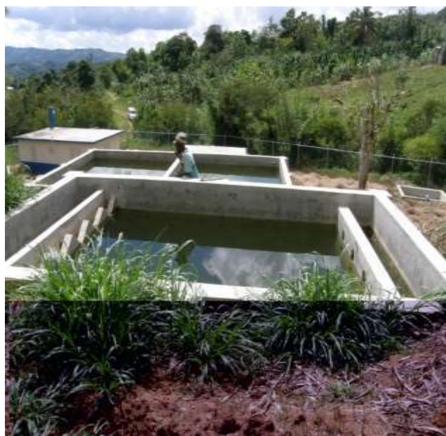
Cascade Water Supply : Settlement Tanks
