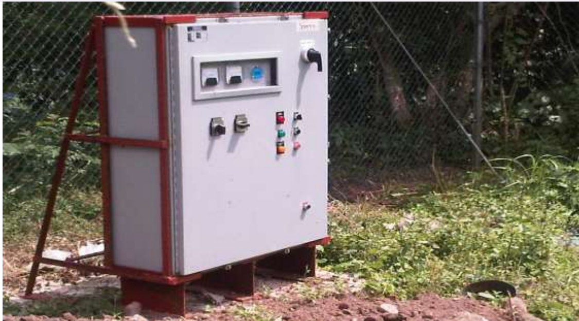
Broadgate Water Supply: - Switchgear for Well Pump
