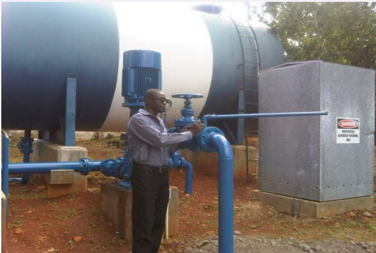
Colbeck Heights / Red Ground / Bartons Water Supply : Pump Station
