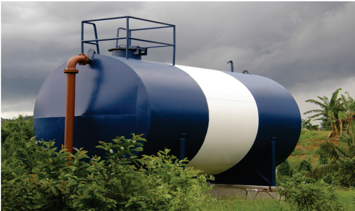
Cascade Storage Tank
