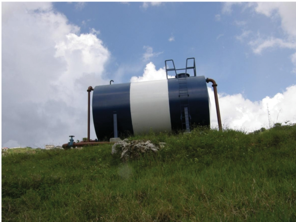
Cascade Water Supply, St Ann - Storage Tank
