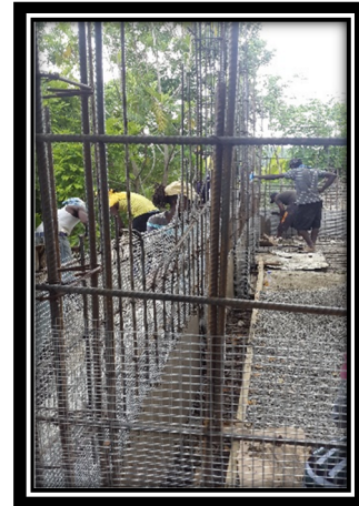
Pear Tree River WSS, St. Thomas – Ferro Cement Tank (Before)
