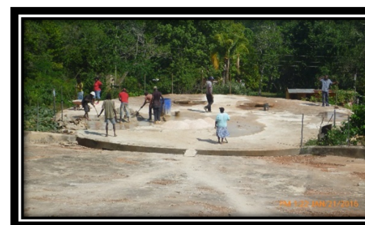
Darlow Rainwater Catchment Tank, South Western (SW) Clarendon – Work being carried out
