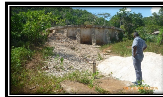
Darlow Rainwater Catchment Tank, SW Clarendon
