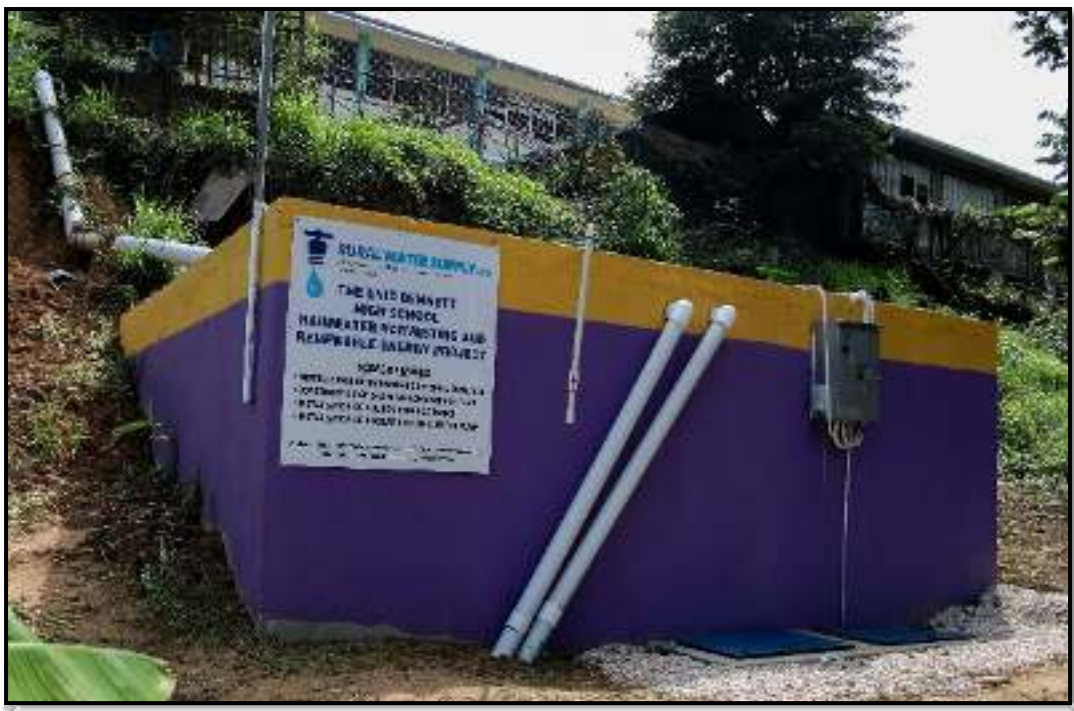
20,000 gal. Storage Tank at the Enid Bennett High School, St. Catherine
