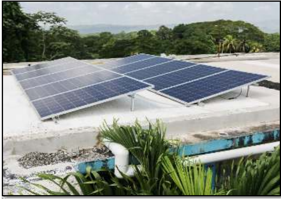
Solar Panels installed at the Enid Bennett High School, St. Catherine
