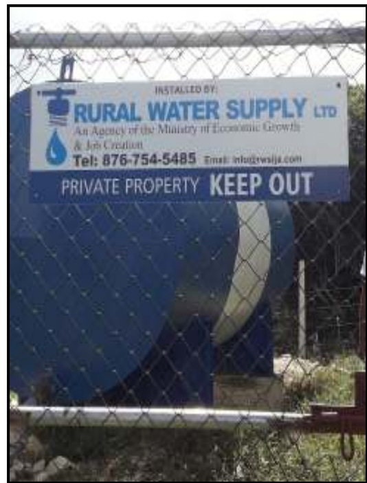
Spring Gardens Steel Storage Tank
